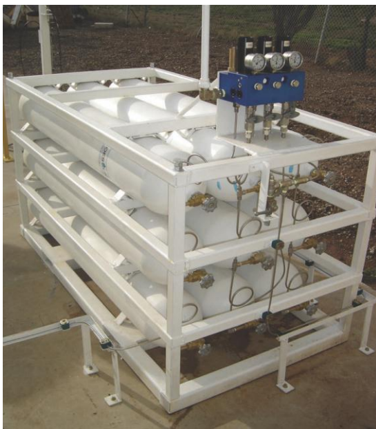
Bulk Storage Bank
